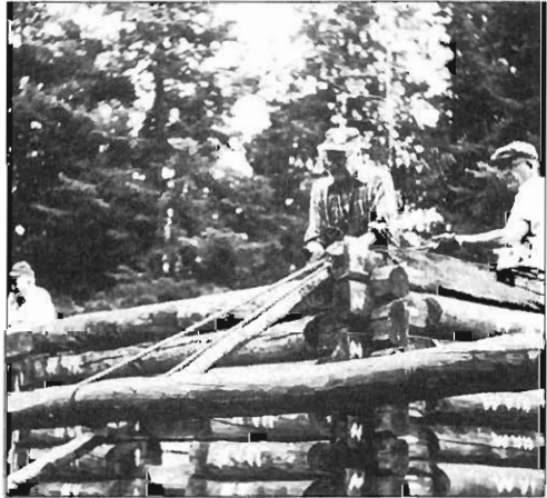
All the timbers were carefully marked at each end, and the weathered tamarack logs were pulled into their respective places. Note the typical Finnish corner notches.
